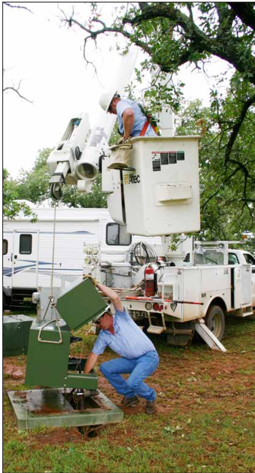
Cotton Electric's Larry Crowell holds the pad mount transformer steady as Bob Anderson guides it into place. Cotton Electric crews spent the first weekend in June restoring power to members who experienced outages as a result of the powerful thunderstorms that blew into the area.
