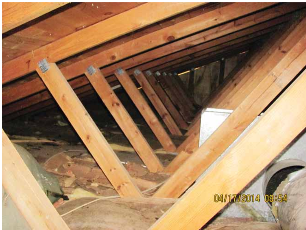
When Mike Stephens, Cotton Electric's energy use advisor, first visited Blaine Smith's attic, he found inadequate insulation and a duct that had been damaged and pulled away from the home's HVAC air handler.
