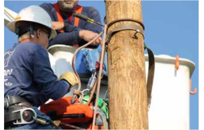
Ely King, Cotton Electric apprentice lineman, works quickly to complete his poletop rescue drill. Photo by Carli Eubank.
